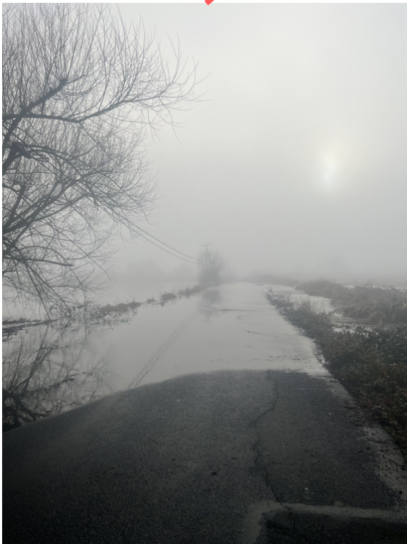
8:20am, turning onto 100 th St., heading east. Water spilling over road from north fields into southern fields where gauge is.
